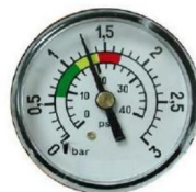
1.3 kg/cm 2 - 18.5 PSI: The pressure is by 0.5 kg/cm 2 higher than the initial pressure, indicating the need for FLUSHING.
